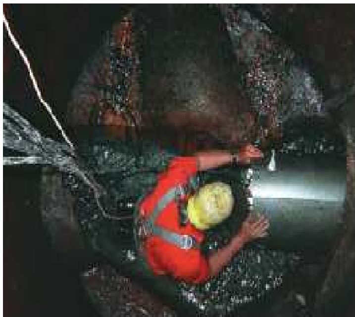
Sleeve installation in sewer. Transducers are pre-mounted on sleeve Model 7510 Multiple-Path Compound Transit-Time Flowmeter
